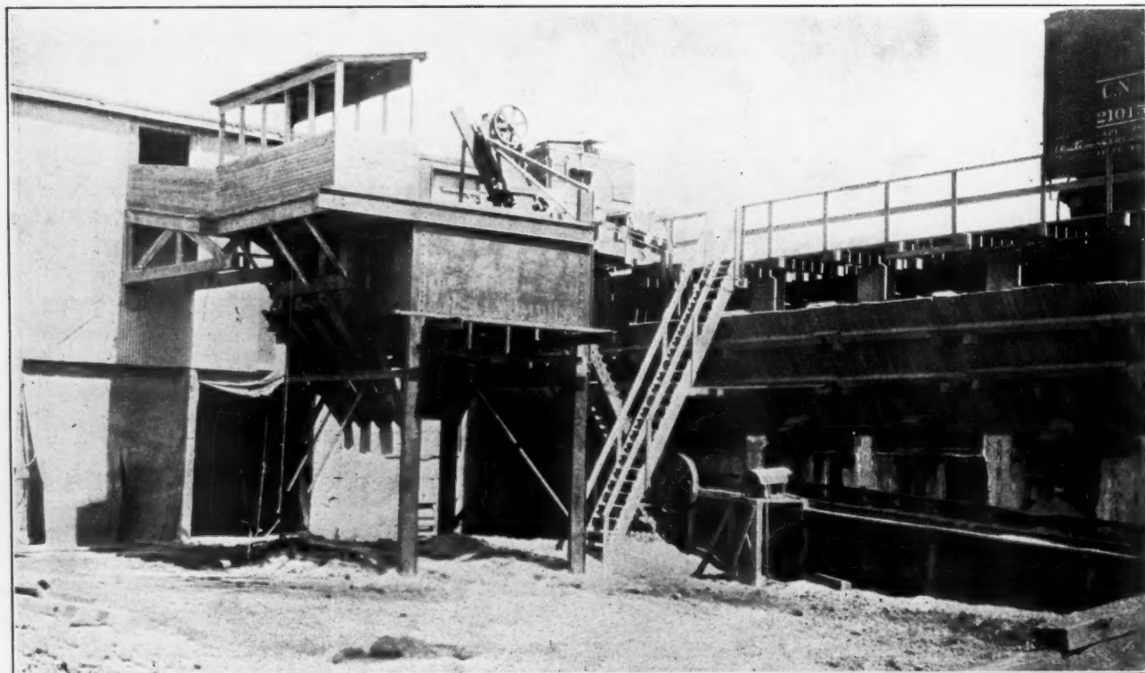
Aggreometer With Conveyor From Under Sand Bins Which Are Below Railroad Tracks
